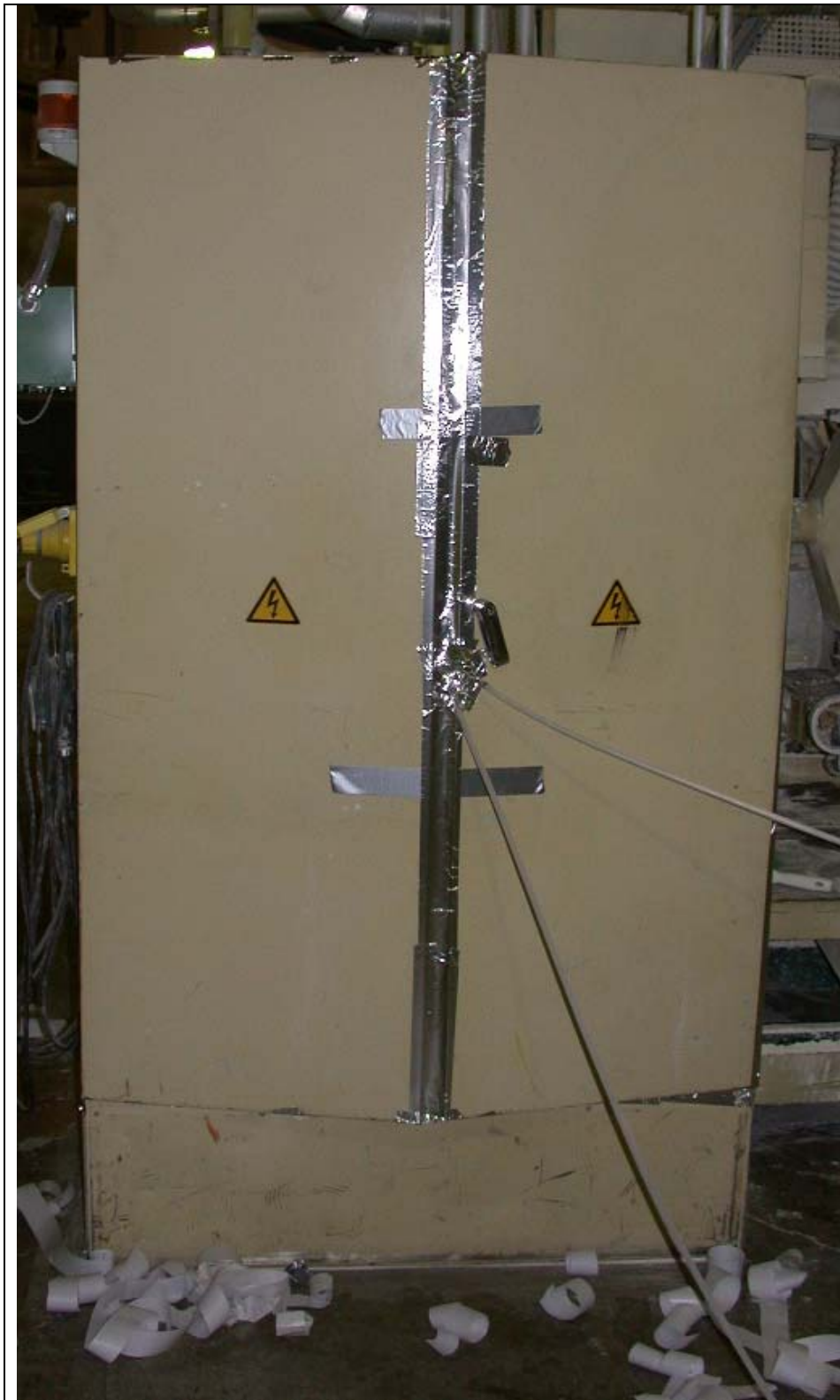
Figure 7. Electrical equipment sealed and pressurized to prevent the entry of phosphine during the phosphine combination treatment, Mill 6.
