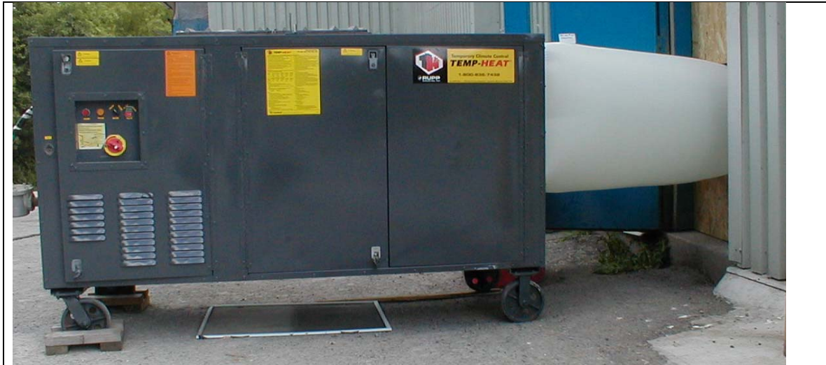
Figure 1. Propane-fired heater (Temp-Air) heating Mills 1 and Mill 7. The door was sealed with plywood, and a flexible fabric duct delivered heated air through a hole cut in the plywood.
