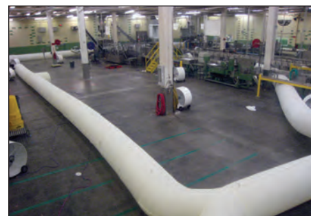
A typical heat treatment installation showing ductwork and fans to distribute hot air and manage the airflow.
