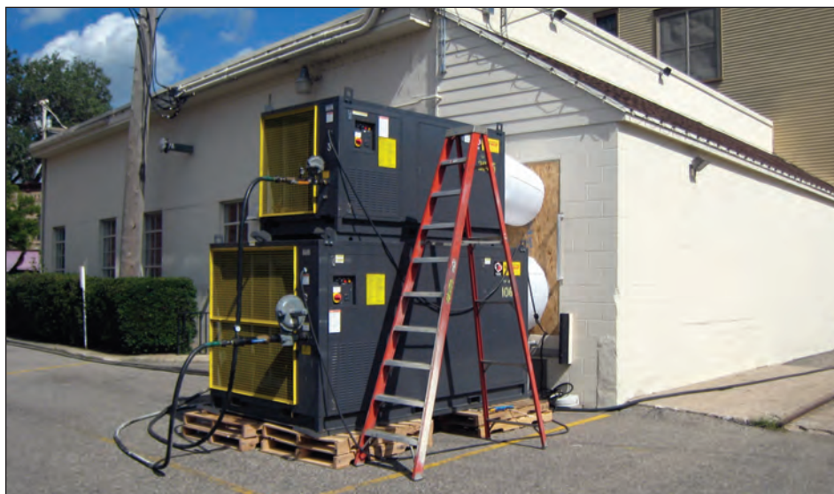
At this facility, a two-tiered heating unit is set up with the proper ducting to deliver enough dry heat during a 24-hour period to control stored-product pests.
