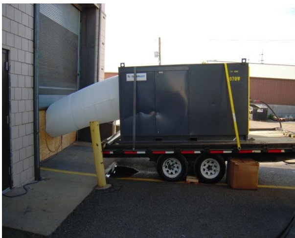
Fig. 3. Heater Placed outside receiving area
